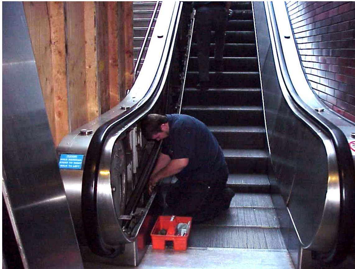
Escalators out of service
