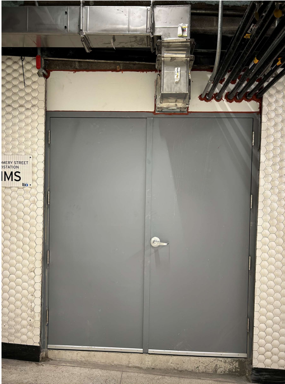
Three Hour Rated Wall and Door at Montgomery Substation
