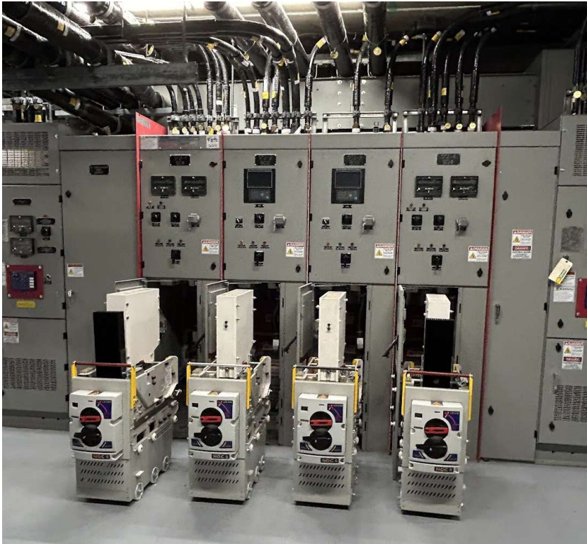
Civic Center Substation Direct Current (DC) Breakers
