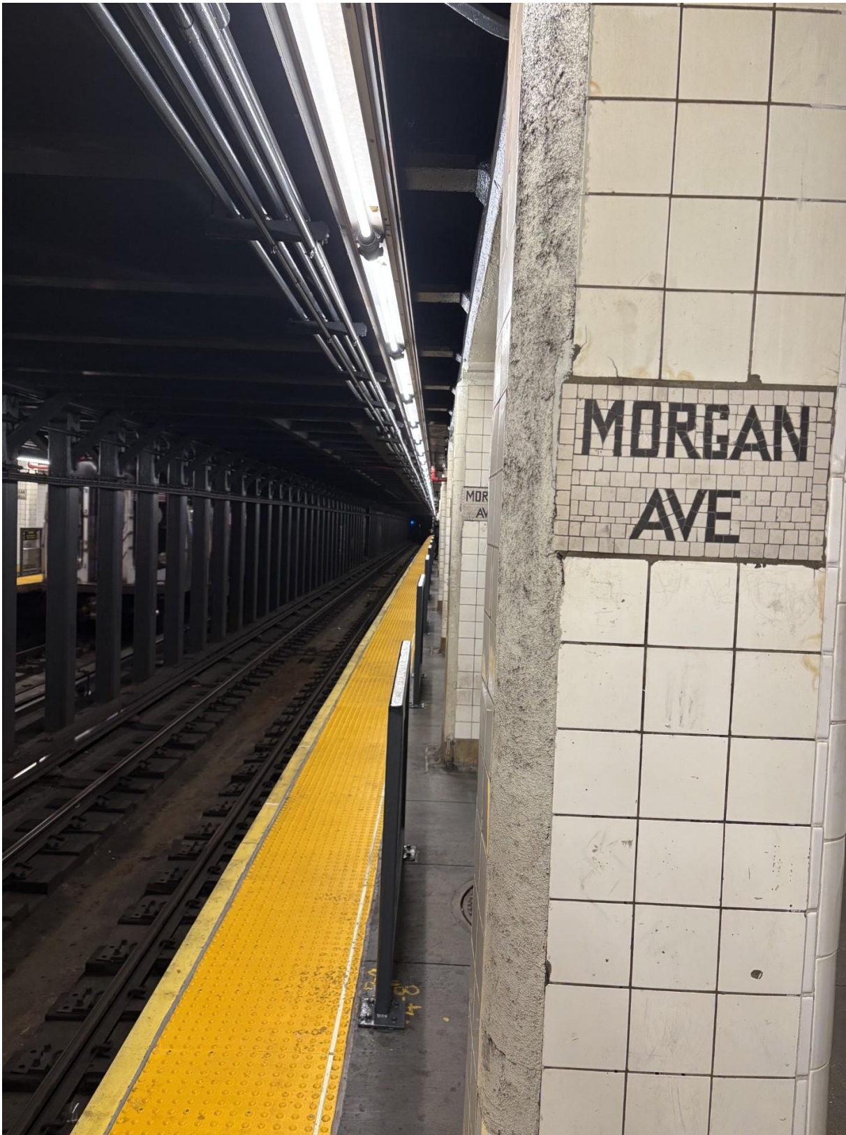
This is the Morgan Avenue Subway Station (L service, B Division, BMT).
