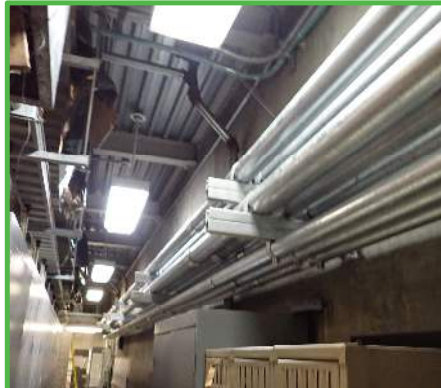
Continued installation of new conduit in the Daily City Train Control Room
