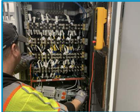
Colma Train Control Room Testing
