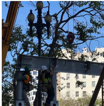
Tree Removal Tree Conflict with Entry Canopy
