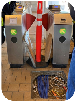
Communication & Power Cables
