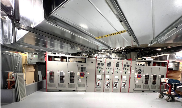
West Bay Traction Power Substations
