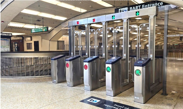
Next Generation Fare Gate Procurement & Deployment
